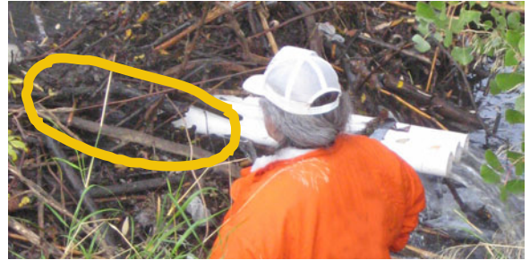
1b) SAVE SOME OF THE DEBRIS YOU REMOVE WHEN YOU CREATE SPACE FOR THE DAM AS YOU'LL WANT TO PLACE DEBRIS ON TOP OF THE PIPES WHEN FINISHED TO REDUCE THE CHANCE OF THE BEAVER ABANDONING THE DAM AND BUILDING A SECOND DAM
