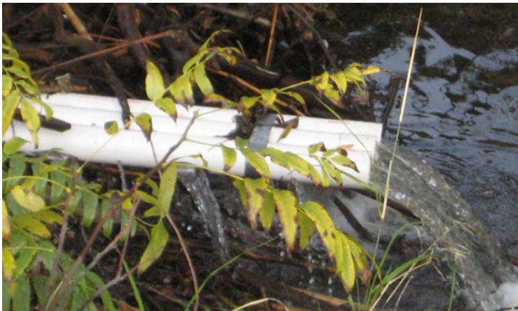
6b) WATER OUTLET SHOULD BE DOWNSTREAM FROM BEAVER DAM
